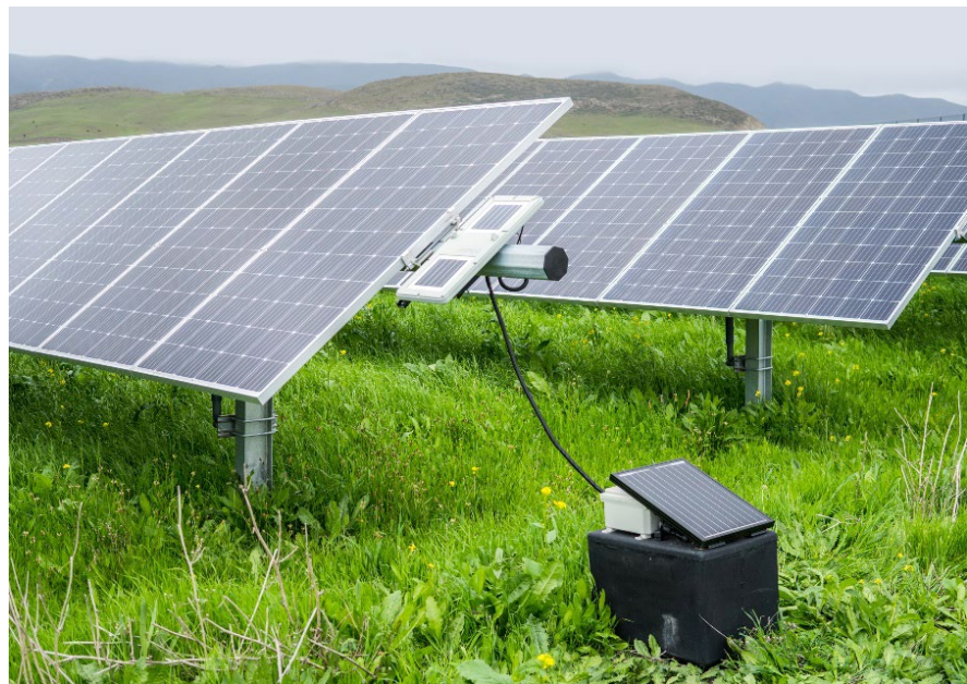
Figure 1: ARES and Wash Extension devices installed within the array
