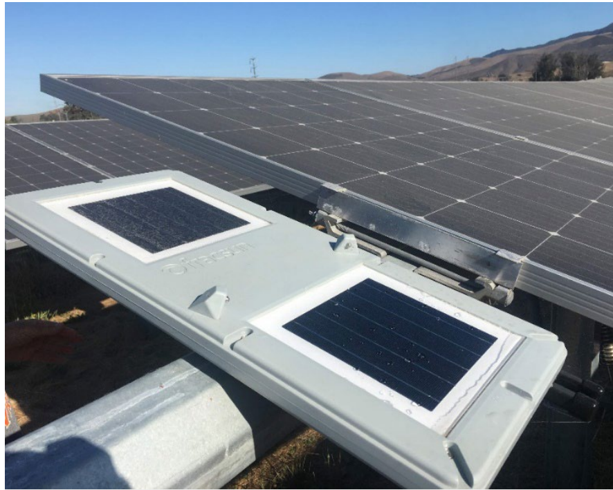
Figure 2: ARES device in the field exhibiting 4% soiling loss
